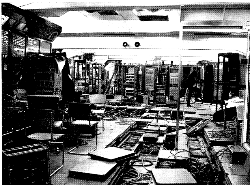
Scene in the main control room of the proton synchrotron during the shut-down. With the development of new techniques in recent years, the adjoining counting room has been used less and less whilst the amount of control equipment for the accelerator has grown. A convenient solution has been found by removing a partition and incorporating one bay of the counting room into the control-room area.
